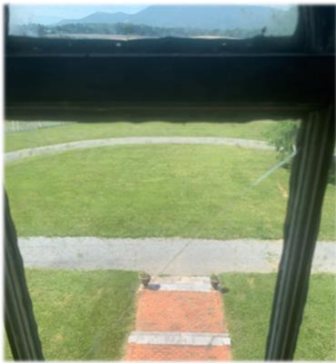
Crack in the portico window
